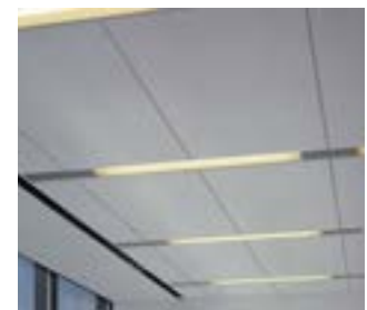
Long Panel Ceiling
